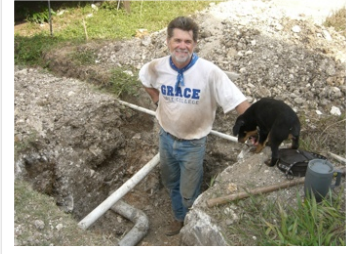
Shaka taking time away from security to "help" with the sewer lines.
